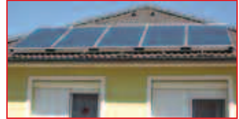
Solar water heating panels
