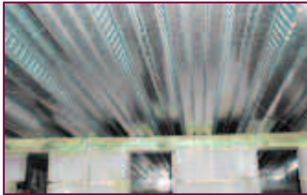
Galvanised steel decking forming the underside of a ground floor slab after 10 years
